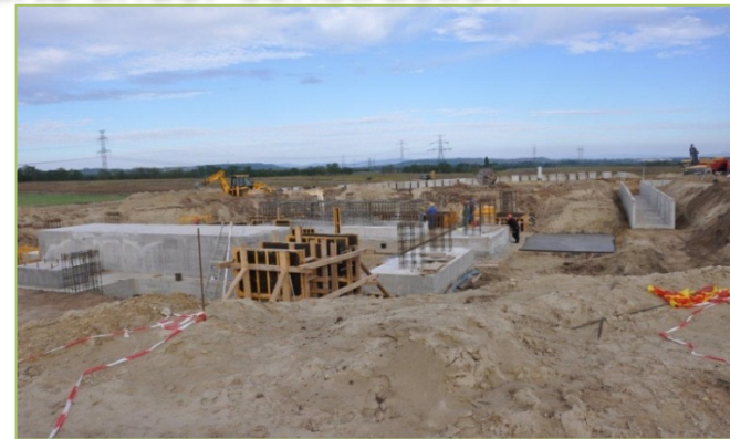
Compressor station at Szada
