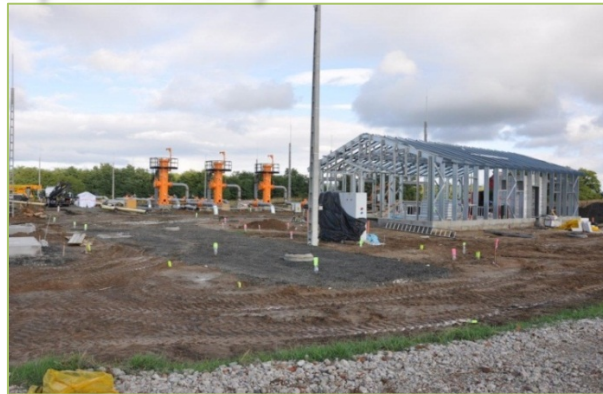
International metering station at Balassagyarmat
